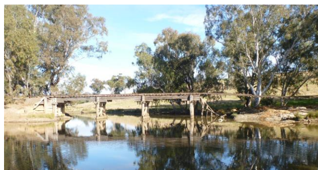
Photograph taken looking upstream at Railway Bridge No. 2 (refer Figure 2.7 for location). Major scour of the western bridge abutment can be seen on RHS of photograph.
