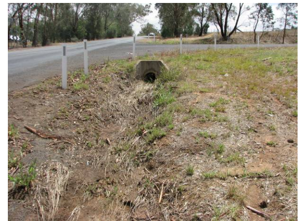
Photo 6: Drainage line on east side may require works.
