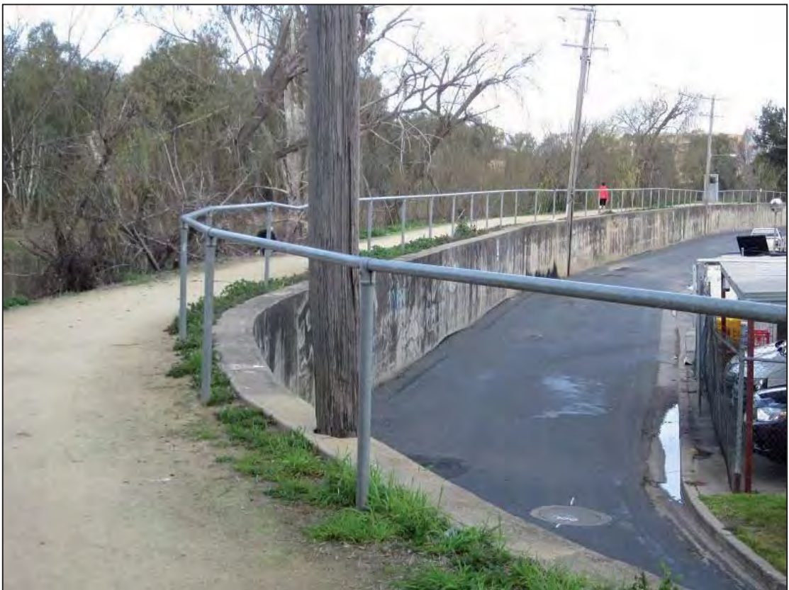
Figure 2.2: Main City Levee - concrete wall levee looking south along Cadell Place, chainage 4500
