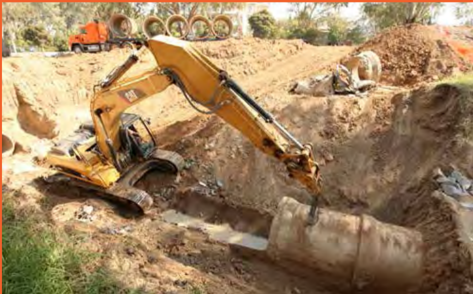
Above: Excavation work to remove damaged stormwater pipes from flood gate 15a, near ARCC Hall on Tarcutta Street, Wagga Wagga.
